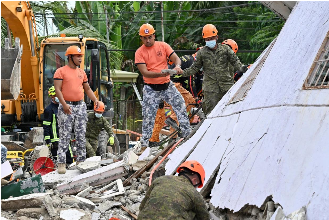
Rescue operations are underway at a collapsed building in Mati City, Davao Oriental, following the powerful 7.4-magnitude earthquake that struck the town on Friday morning, October 10, 2025. (Photo courtesy of NBC News via online)
