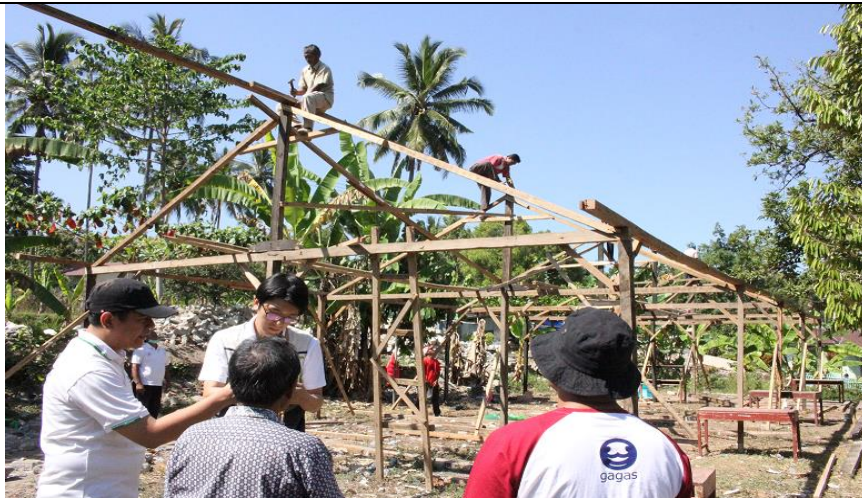
Temporary school construction by community which will use as well for CCS center
