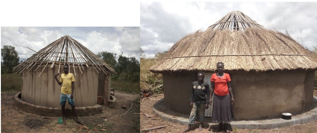
Above: Progress on reconstruction of houses for people displaced by floods in Lango region in Northern Uganda.
